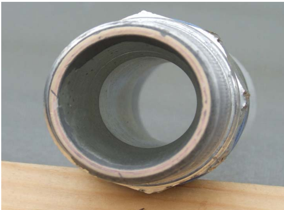
Discharge side into commissioning station
